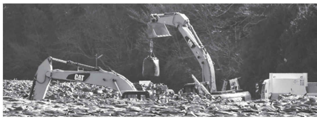
Excavators piling nuclear contamination at a temporary place in Tomioka, Fukushima prefecture.
